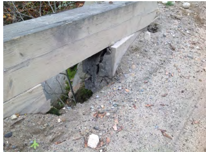
damaged riser and block
