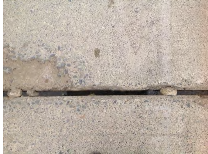
missing all deck joint seals
