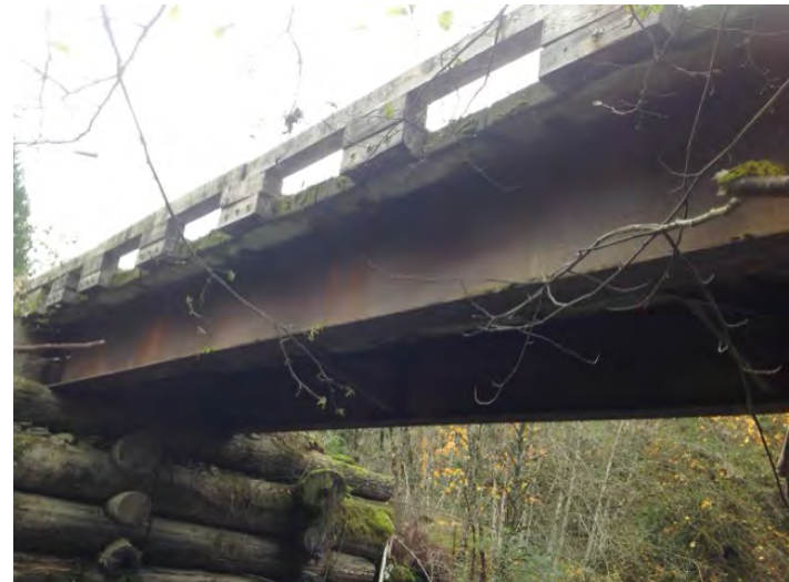
missing and loose deck clips
