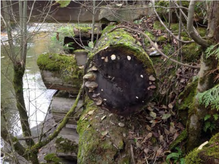
Douglas Fir sills starting to deteriorate
